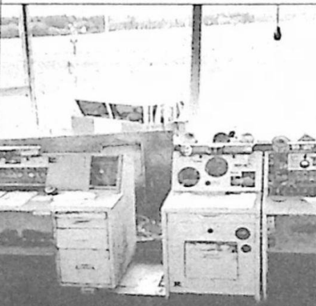
The tower is prepared for an equipment update in the 80's. Note the mobile control tower in the background.
