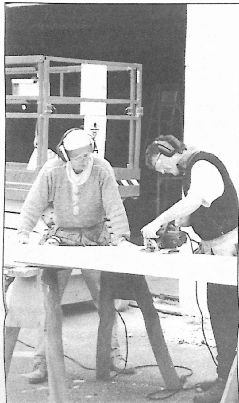
CE's Lance Callera and Charles Turner cutting covering before overhead door installation.
