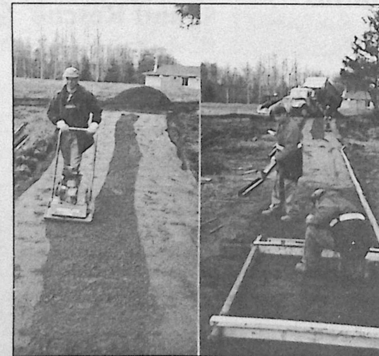
...and John Egan and Deavlan Bradley prepare the rails that will frame the concrete.
