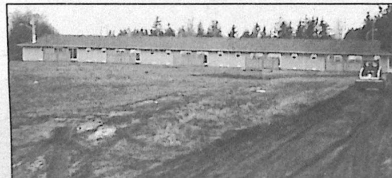
Path being levelled by Norm Maximick in front end loader while Dave MacDonald smoothes dirt...
