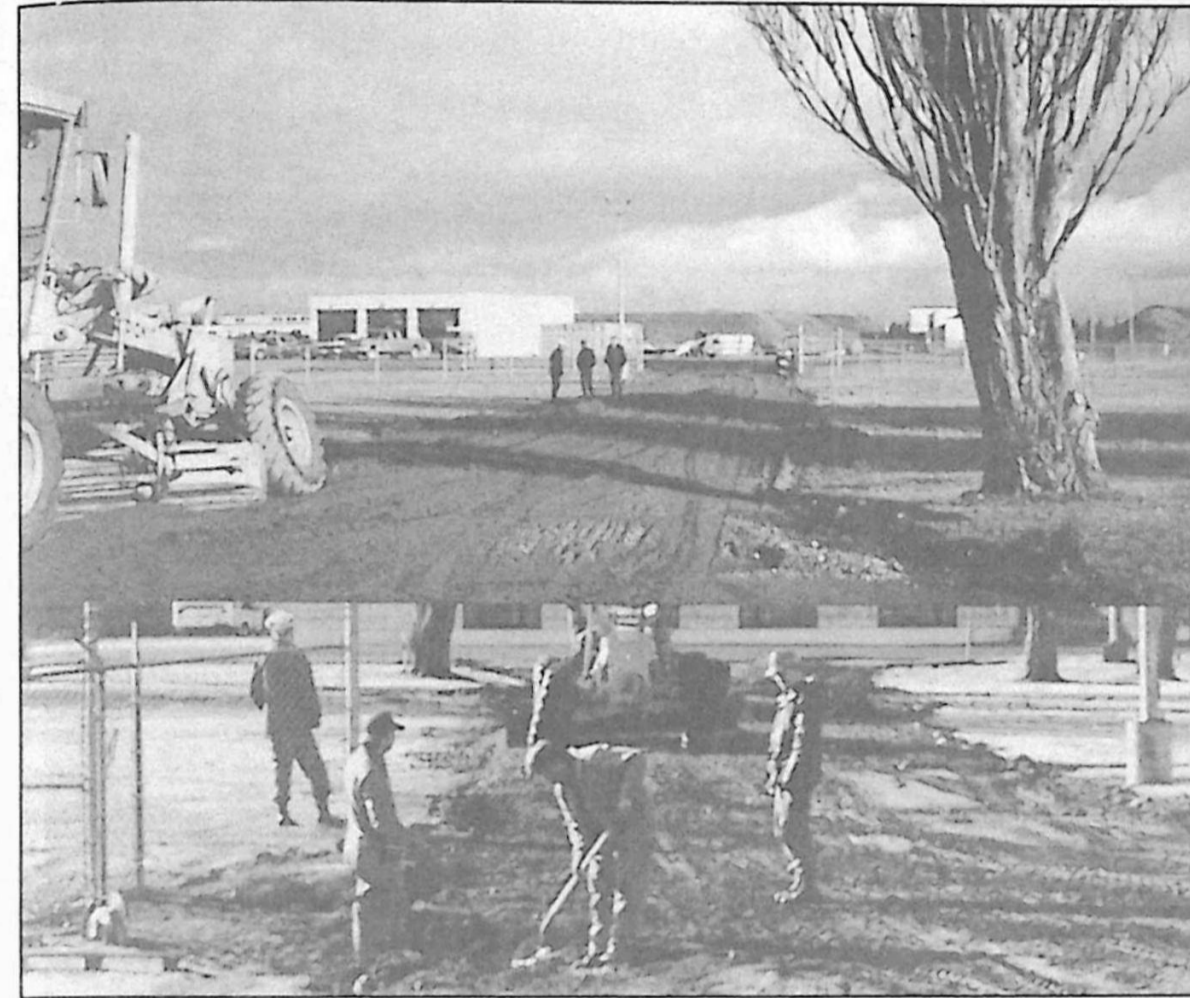
The road builders: personnel from W Tn flank CE's Norm Maximick (L) and John Egan.
