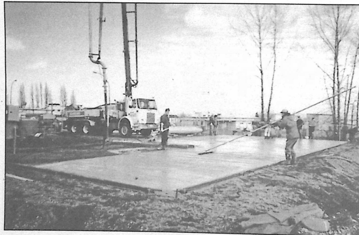
Construction Engineering crew hard at work pouring the new pad for the hangar of the Heritage Aircraft Restoration Committee. The hangar will be erected on the new site once the surrounding fields dry out a bit.
