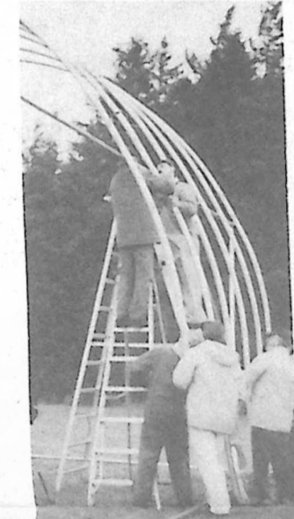
Temporary hangar being erected by the Heritage Committee volunteers, with technical assistance provided by Capt Bob Richter.
