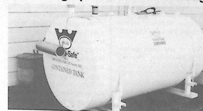
A new double-walled fuel storage tank has been installed at the Water Pumphouse Building. (Photo by Cpl Kelley)
