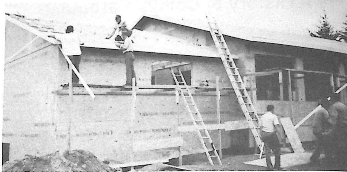
All-volunteer crew applies sheathing and roofing to the Wing building, airfield side
