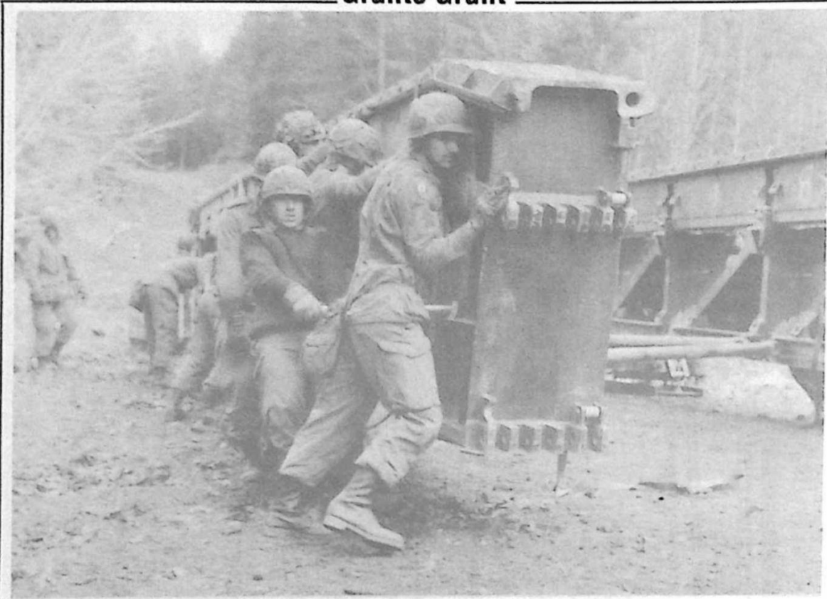
SAPPERS from 2 Troop, 1 Canadian Engineer Regiment based at CFB Chilliwack dismantle a medium girder bridge while on Exercise Valley Run 88.
