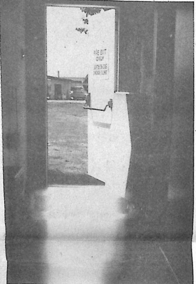
How it looked to the accident victim, just before falling bodily through the trap, onto the access ladder, a fall that could have been fatal.
